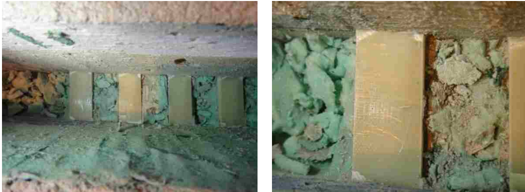
Figure 70: Post-failure examination of exposed shear tie legs
